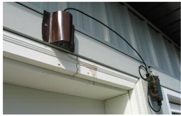
Trail counter installed over the kitchen door at Broad River Multi-Use Compound Credit: Doug Clark
