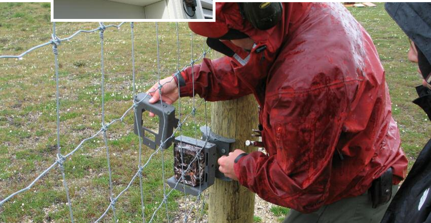
Doug Clark installing the protective case over a remote camera Credit: Parks Canada
