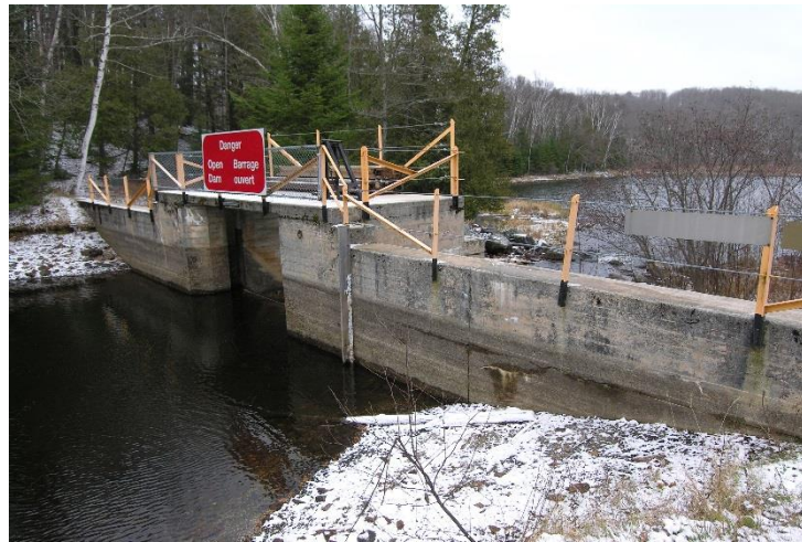
Loon Lake Dam Prior to Repairs
